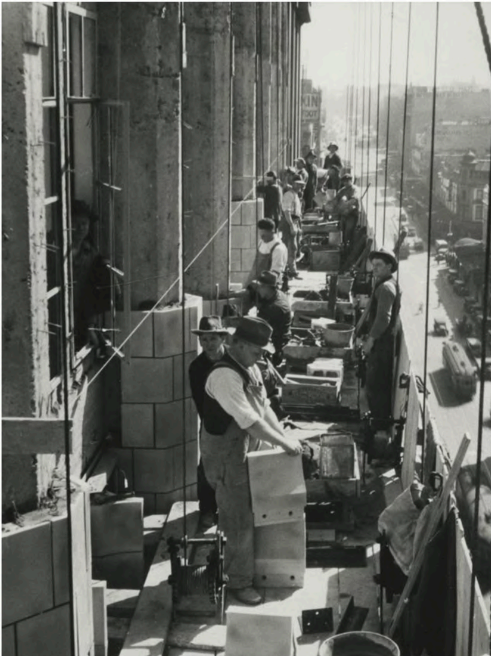
📷 Labourers on the east side of the Manchester Unity Building in 1932. Work continued around the clock. Picture: University of Melbourne Archives
